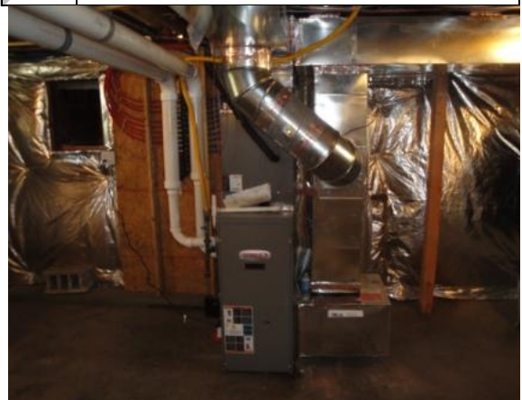
Photo #6 New Natural Gas Furnace and Air Handling Unit
