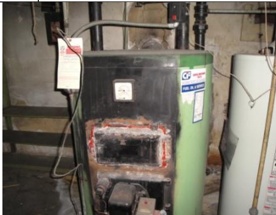
Photo #3 Pre-Renovation Oil Boiler
