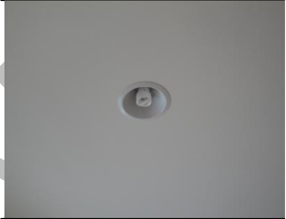
Photo #10 New CFL Recessed Lighting Fixture
