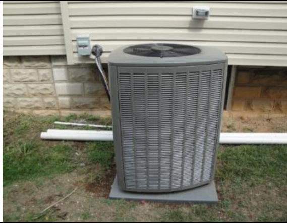
Photo #9 New Ground Mounted Exterior Condensing Unit
